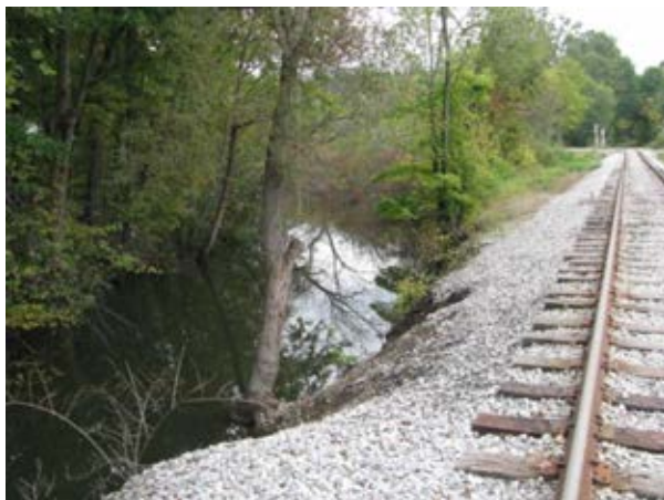
Photo 37: Stream Bank Issues (looking south)
